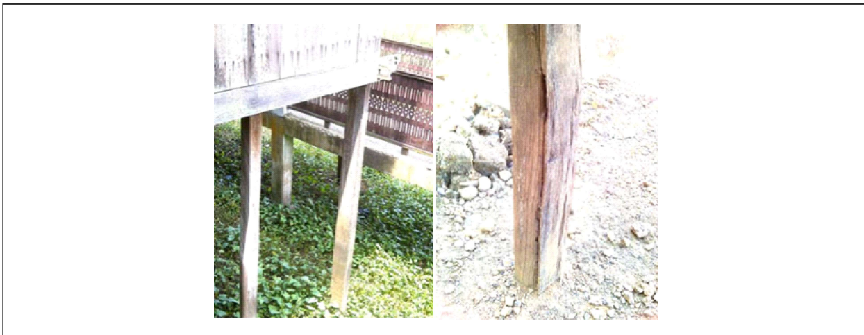
Figure 2: Damage to Wooden Pillars
