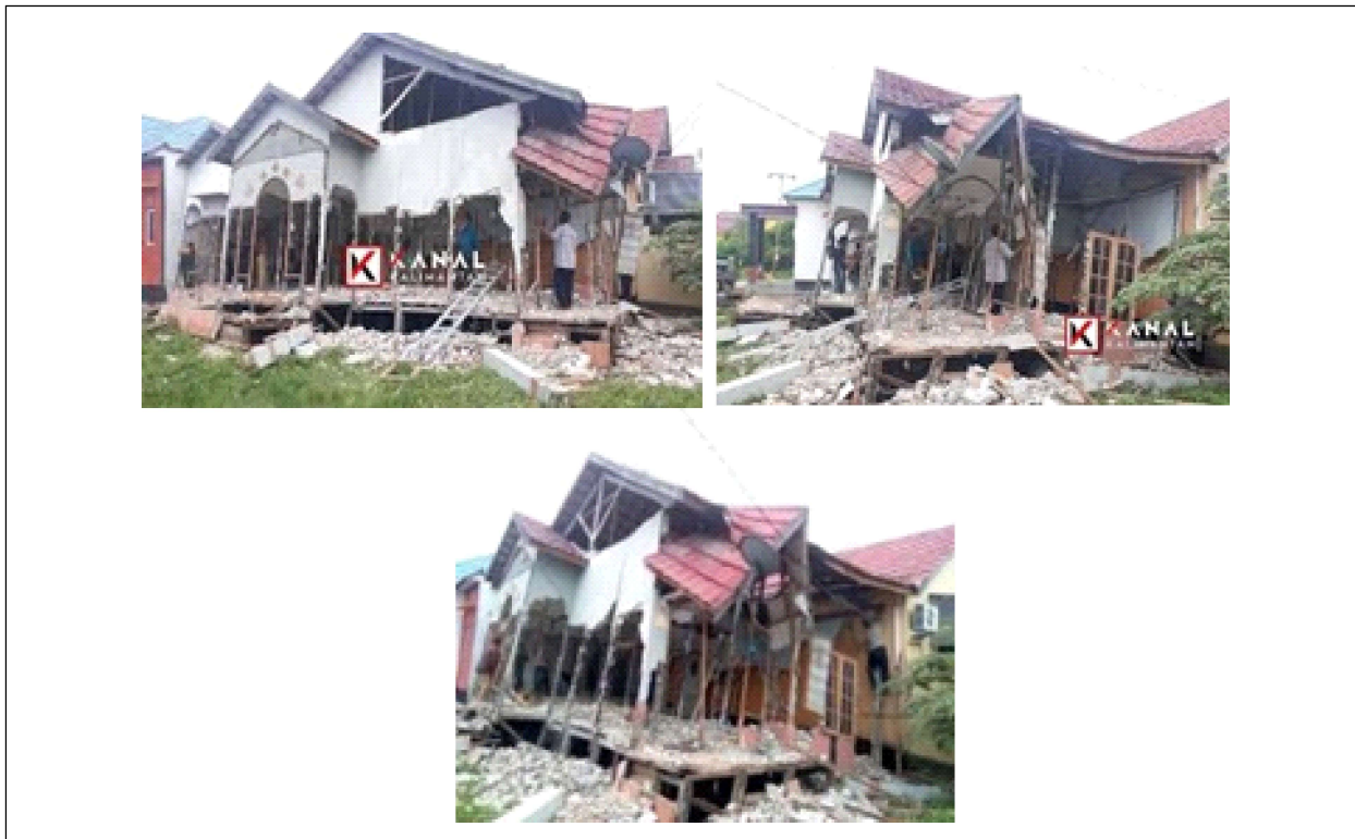
Figure 12: Tilted House Building
